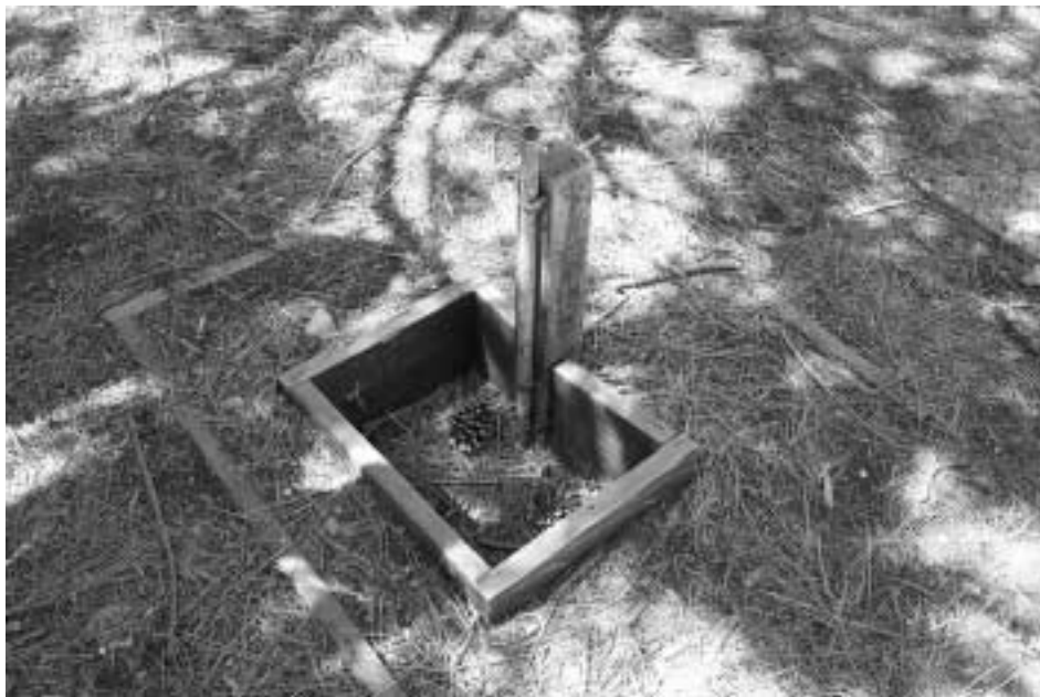
Photo 6. Well at abandoned faucet in Canyon Dam picnic area was filled in after the inspection to assure public safety.
