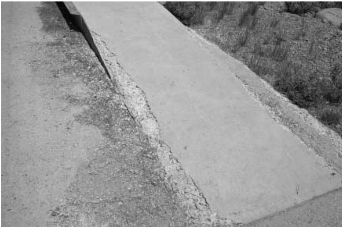
Photo 20. Spalled concrete at the Almanor Campground boat launching ramp.
