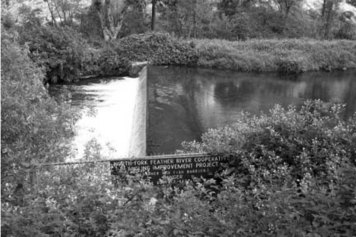
Photo 3. Gansner Bar Dam with warning sign partially obstructed by berry bushes (the licensee removed the vegetation for a clear line of sight after the inspection).
