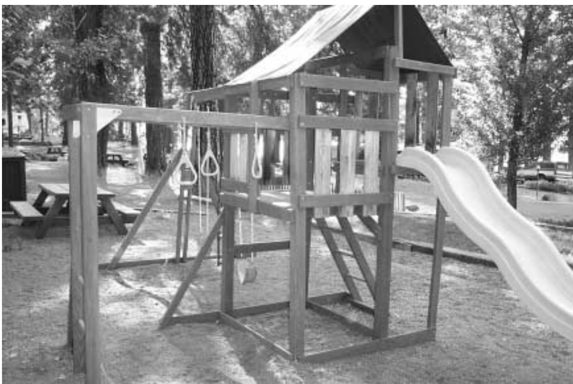
Photo 10. Child play structure at Northshore Campground had loose connections, sharp edges, and exposed bolts. It was removed after the inspection.
