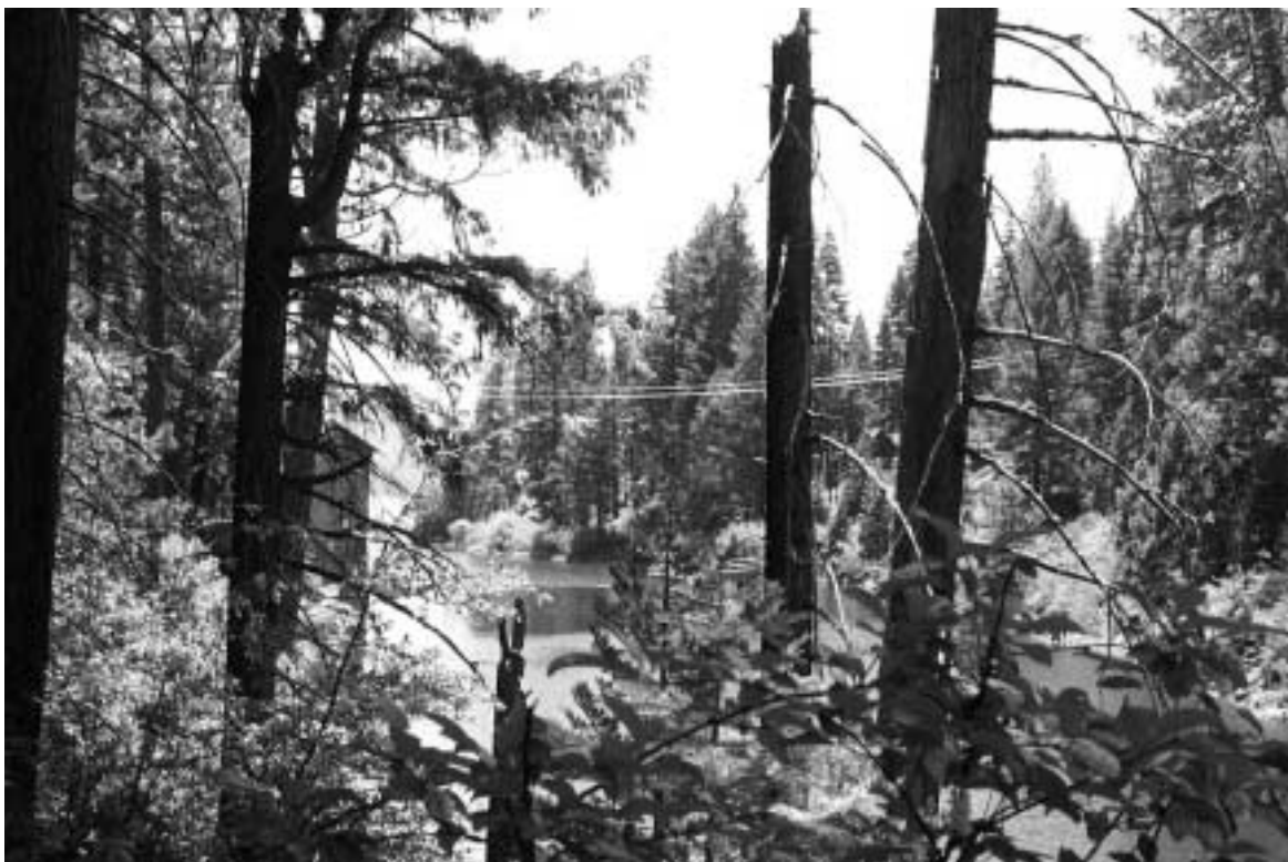
Photo 15. Transmission line crossing at Hamilton Branch Arm of Lake Almanor Reservoir is reported to meet NESC clearance requirements.
