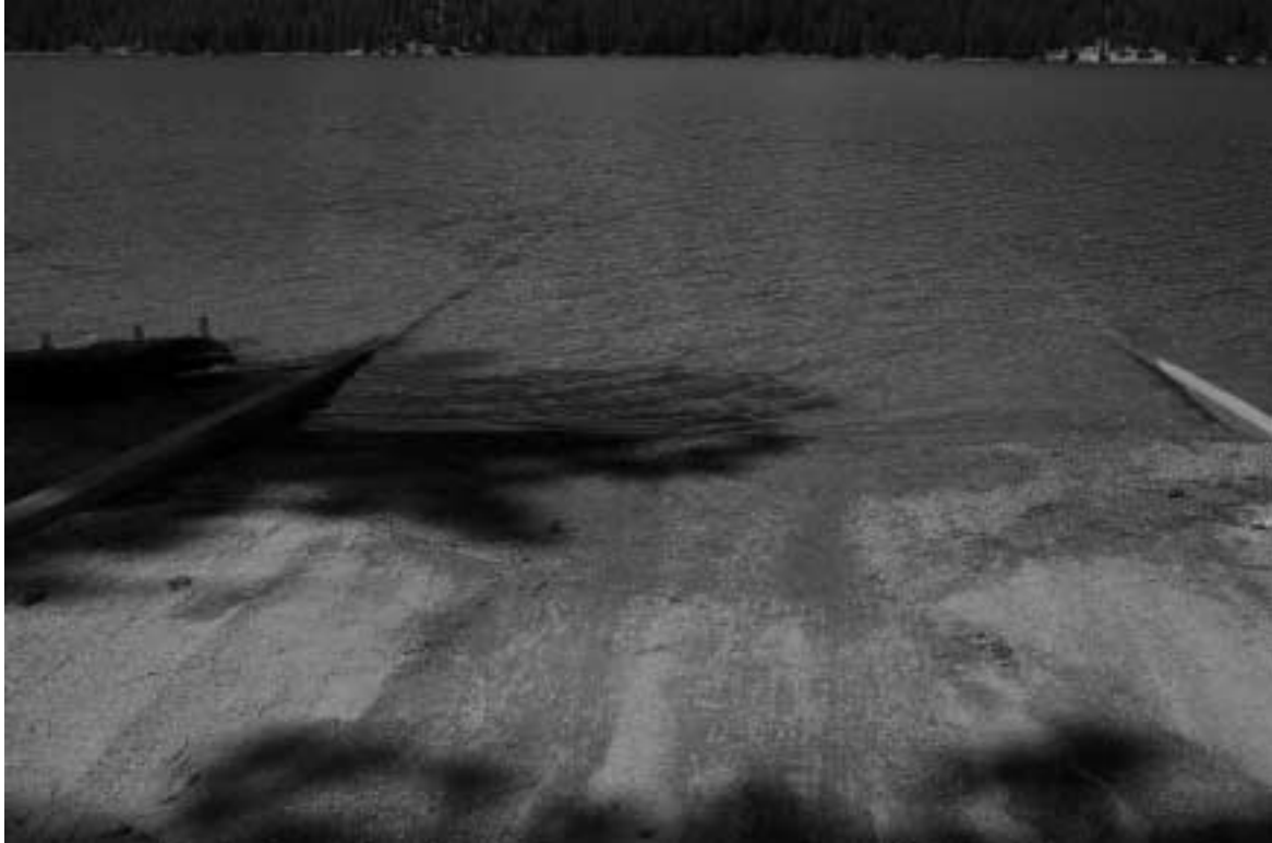
Photo 19. Sediment on the Alder Creek boat launching ramp was removed after the inspection.
